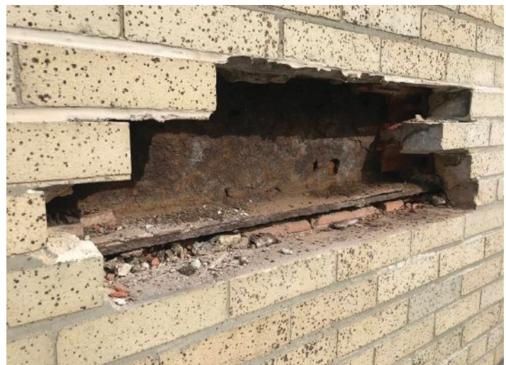
Test cuts can provide insight into the existing layers, securement methods, and material conditions.
