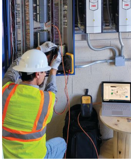
Methods for monitoring and maintaining our buildings have changed and become better.
